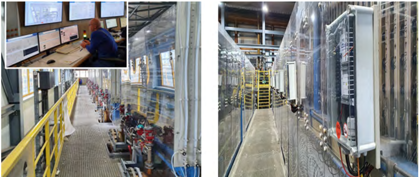
→ Figure 6: Bank of 8 electrolyzers at Nobian's chemical facility, Höchst, Frankfurt
