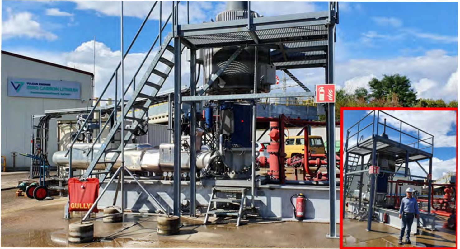
→ Figure 4: Geothermal production well (Amati fund manager for scale)
