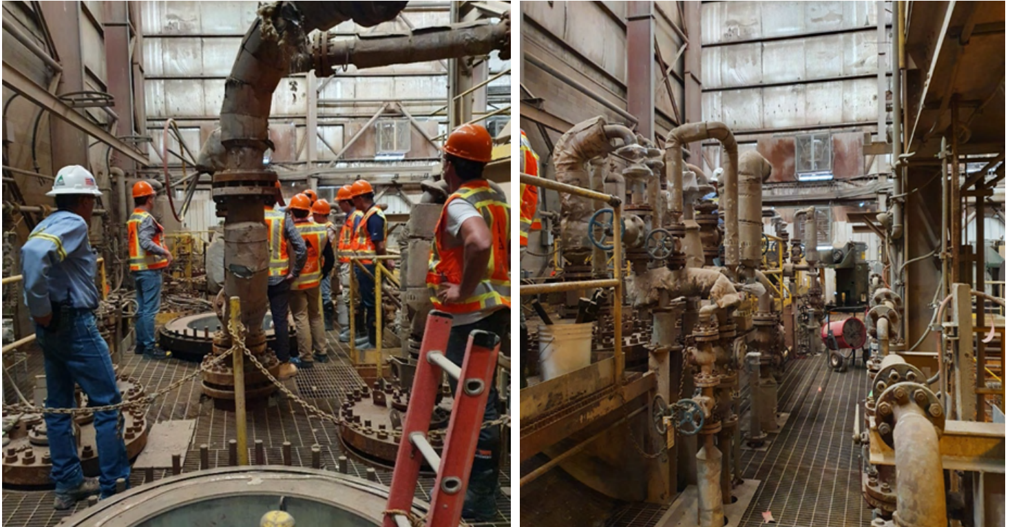
Note the inspection ladder down into autoclave interior. Source: Amati
